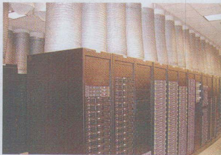
Figure 6: High-density containment systems installed in data center.
